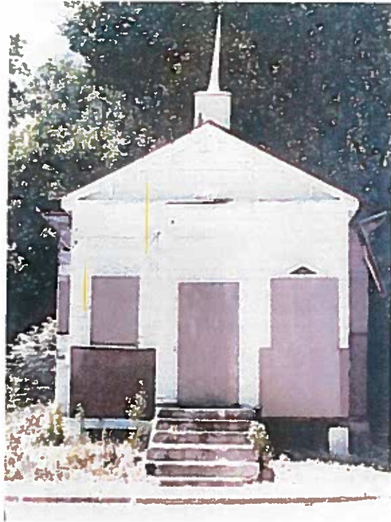
Figure 19. 9 Dereef Court, c. 1988. (Photo from Board of Architectural Review files, City of Charleston Urban Design & Preservation Division)
